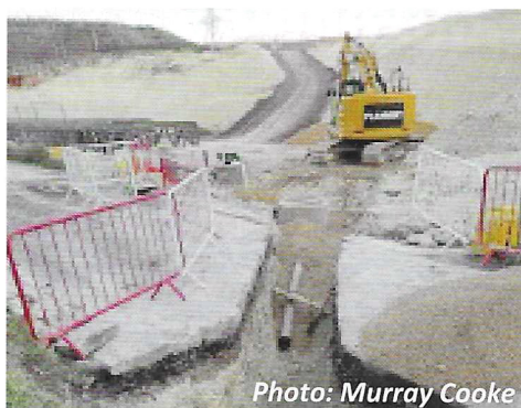
Left: The sewer at Ellesborough Road – a small pipe that played a big part in the construction delay.
