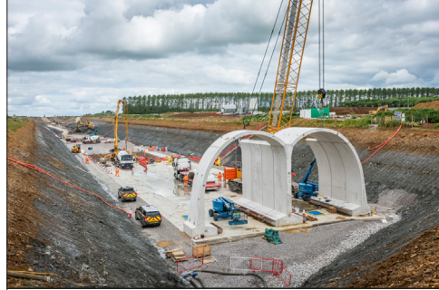
above - Ellesborough Road demolition and EKFB's first green tunnel at Chipping Warden.
