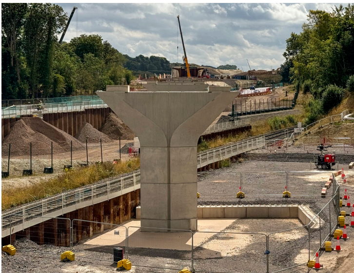
This photograph, taken in August 2024 from the top of the most northerly pier in the series, shows the route that the viaduct will take across the road and railway. The yellow crane boom (centre, top) indicates where the viaduct sits, ready for its ultimate journey.
