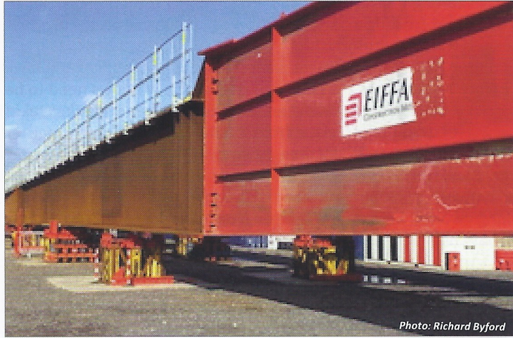
The brown steel part (main beam), will eventually be 350m long for the viaduct nearest Wendover.
