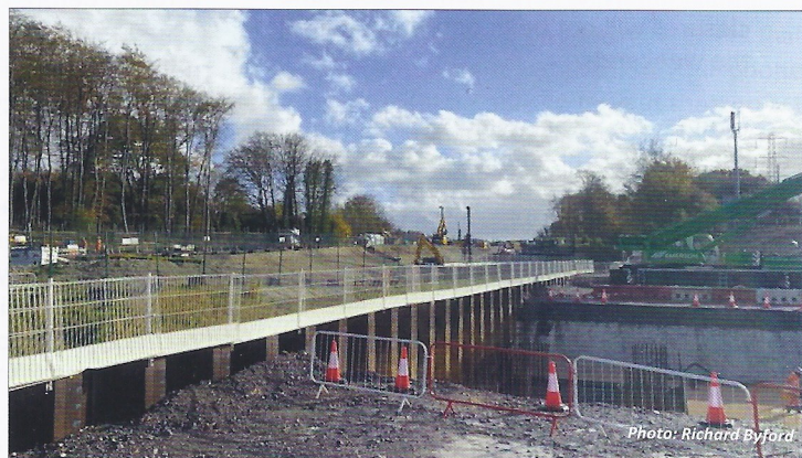
Closer to home, just as you leave Wendover on the A413, this is the view from the 'other side' of the railway. The two pieces of equipment sticking up in the middle of the shot show the route that the completed viaduct will take.
