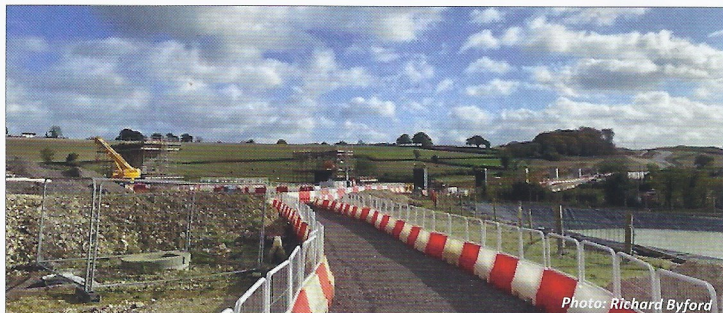
An on-site view of the Small Dean viaduct supports. At the moment, they are hardly visible, when completed, they will just be visible from the London Road.
