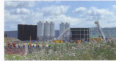
Artist's impression of the second concrete plant to be constructed near Nash Lee Road
