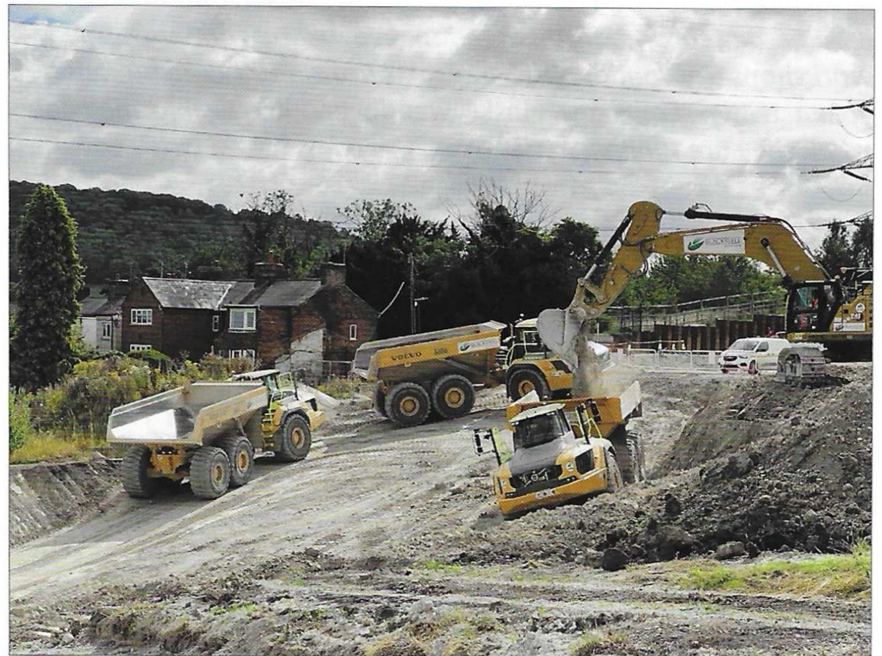
Excavating the haul road ramp at Ellesborough Road: The view is from the new bridge towards Pound Street, and the digger is where the cottages used to be.
