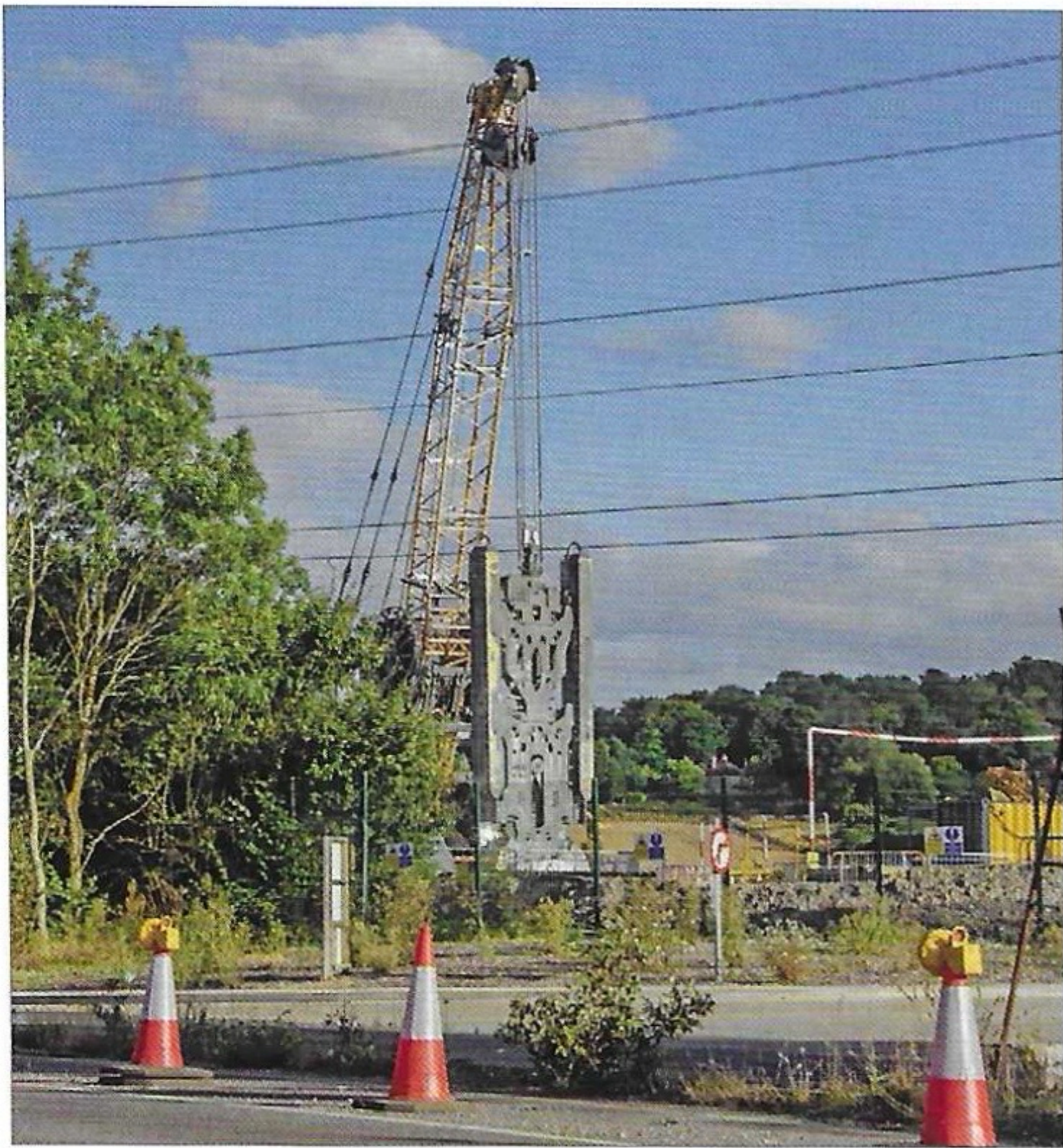
The computerised mechanism of the clamshell excavators enable them to dig very precisely to depth required for the underground wall at the green tunnel
