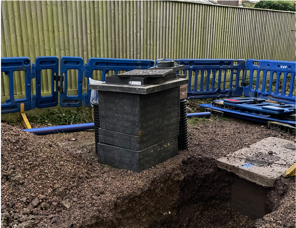
Prefabricated Chamber by Thames Water 15 th Jan '25 at Bridleways. This did not need 150 trucks.
